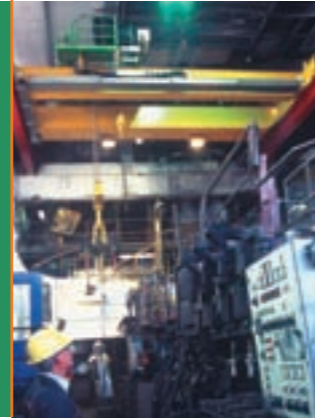
The double girder bridge crane transporting molten metals.
